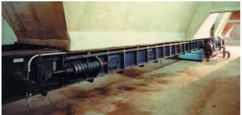
Hopper discharge with armoured chain conveyor
